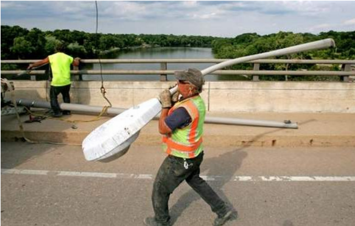
Peter Isherwood carries a street lamp Tuesday as he and Elmstar Electric Corp. co-worker Larry Van Den Heuvel work on the College Avenue bridge in Appleton. Preparations are under way for the structure's demolition beginning Monday. Post-Crescent photo by M.P. King
